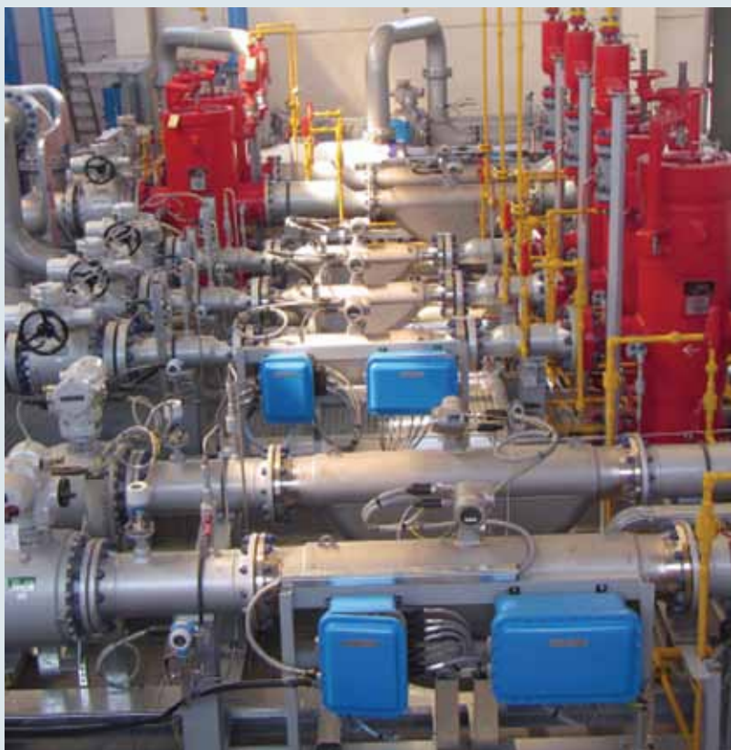
Skid multi – stream, fornitura chiavi in mano
